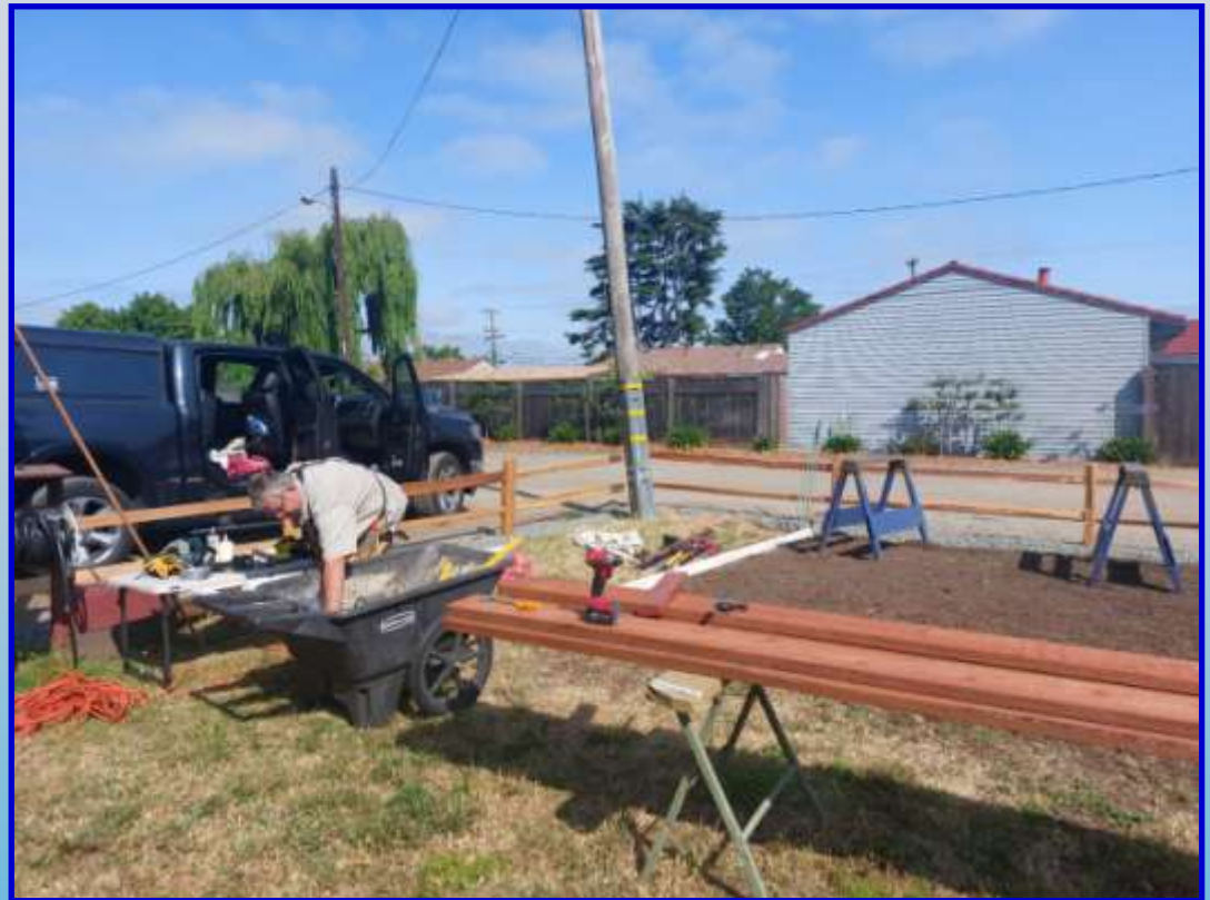
Cris setting up his supplies and equipment for the installation of the wood perimeter border
