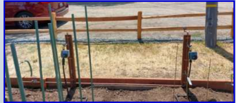
Two Timers Installed
